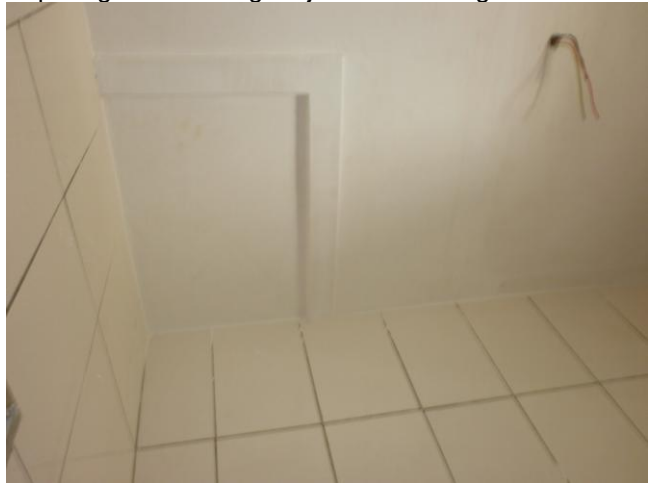
plafondluik in toilet nurses station
